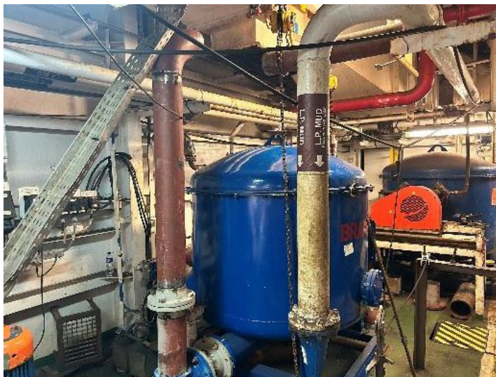
Figure 9 — Existing vacuum degasser vessels in-situ prior to removal, showing LP Mud system piping and surrounding equipment layout
